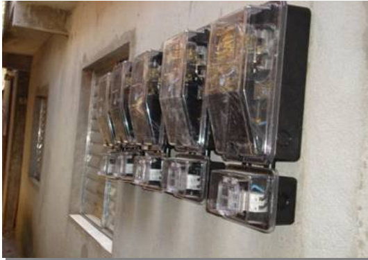
Conventional Meters enclosed in plastic to deter tampering
