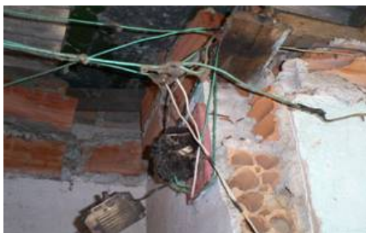
Typical wiring prior to upgrade
